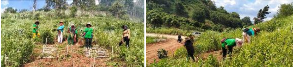
Figure 107. Practicing Maintenance and Replacement of Grass and Live Sticking at Dontret Community
